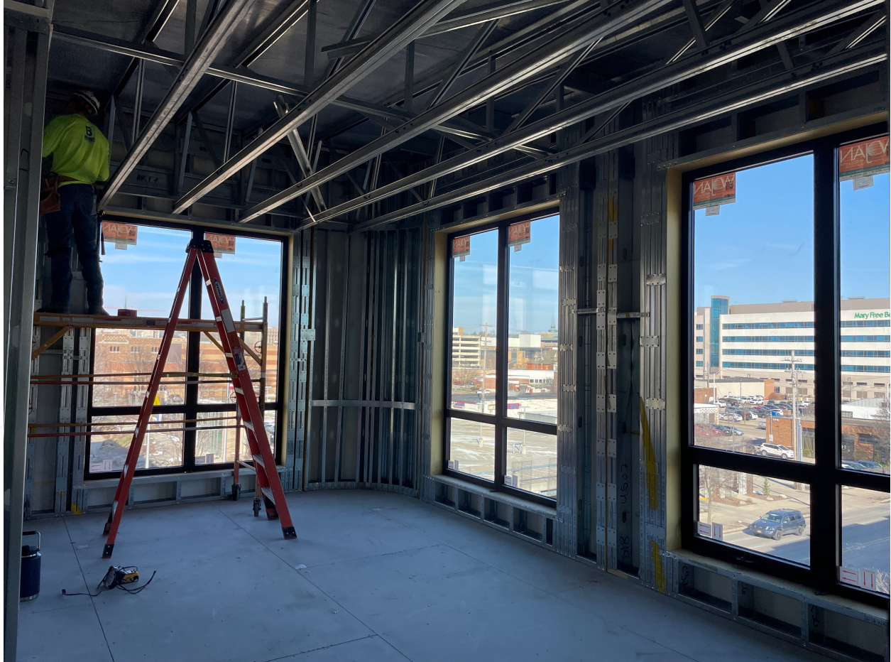
Cella Building Company broke ground last fall on the 58-unit Wealthy & Sheldon Lofts project at 415 Sheldon Ave. SE in Grand Rapids. Credit: Courtesy of Mike Coyne
